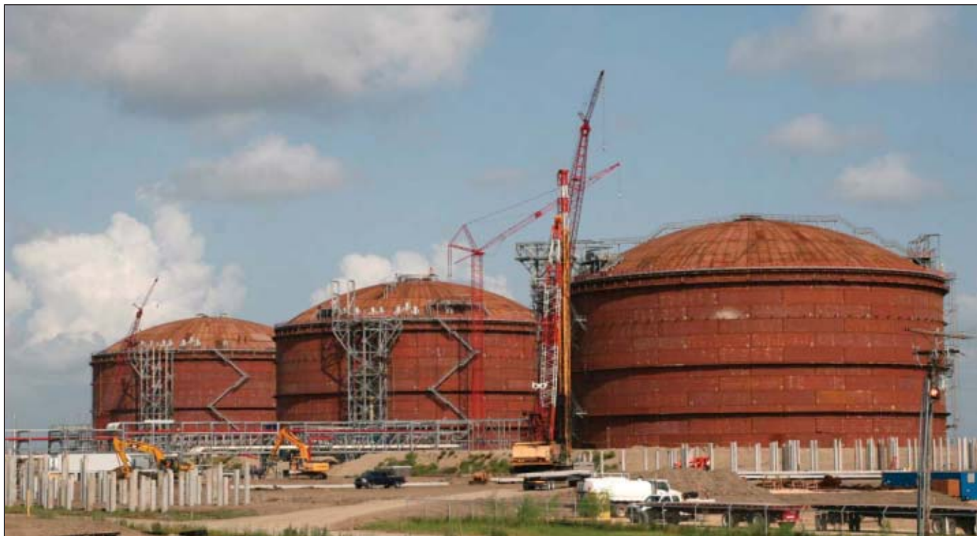
In early August 2007, construction teams raised the roof on a third LNG storage tank at Cheniere's Sabine Pass LNG regasification terminal in southwest Louisiana. These three tanks, of six to be finally built, will have 10.1 bcf of LNG storage capacity. The terminal will begin operations in second-quarter 2008 and have total regasification capacity of 4 bcf when construction ends in 2009. Photograph from Cheniere Energy Inc. by Mike Kelly.
