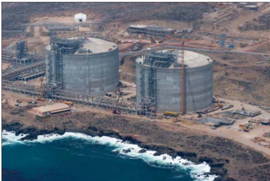
The first LNG regasification terminal on the western coasts of the Americas will open later this year or in early 2008. Semptra LNG's Energía Costa Azul in Baja California, Mexico, shown here in August more than 80% complete, will initially be able to send out as much as 1 bcf/d of Pacific Basin-produced natural gas to Mexican and US markets. Photograph from Semptra Energy.
