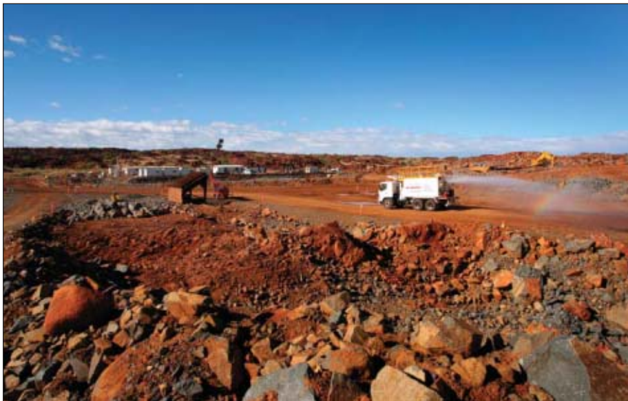
Ground clearing progresses in earnest near Karratha on Western Australia's Burrup Peninsula for Woodside Petroleum Ltd.'s Pluto LNG project. In mid-2007, the company announced it was moving ahead with the 4.3-4.8 million tpy, $12 billion (Aus.) project. Photograph from Woodside.
