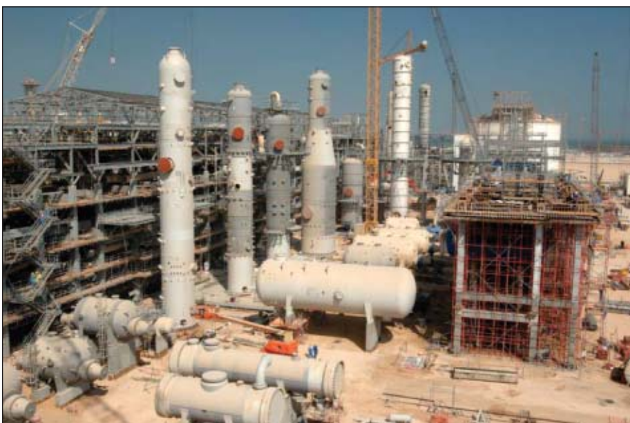
Work progresses earlier this year on the Qatargas 2 expansion project, a joint venture between Qatar Petroleum, ExxonMobil, and Total. The company calls it the world's "largest integrated LNG project from wellhead to customer" and says it will start up next year. When fully operational, Qatargas 2 will supply up to 16 million tonnes of LNG to Europe, mainly to the UK, says the company. Photograph from Qatargas.
